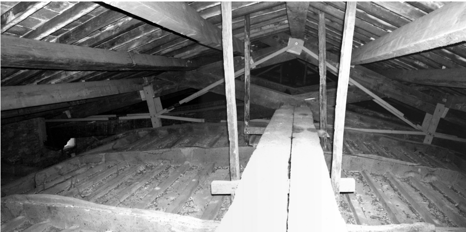
Fig. 8. San Giovanni, Florence: general view of the roof (photograph Hermann Schlimme/Jens Niebaum).
